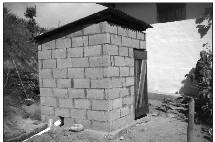
All 40 of the latrines used the same basic design with modifications according to the preferences of the owner. Photos- Linda Wan
